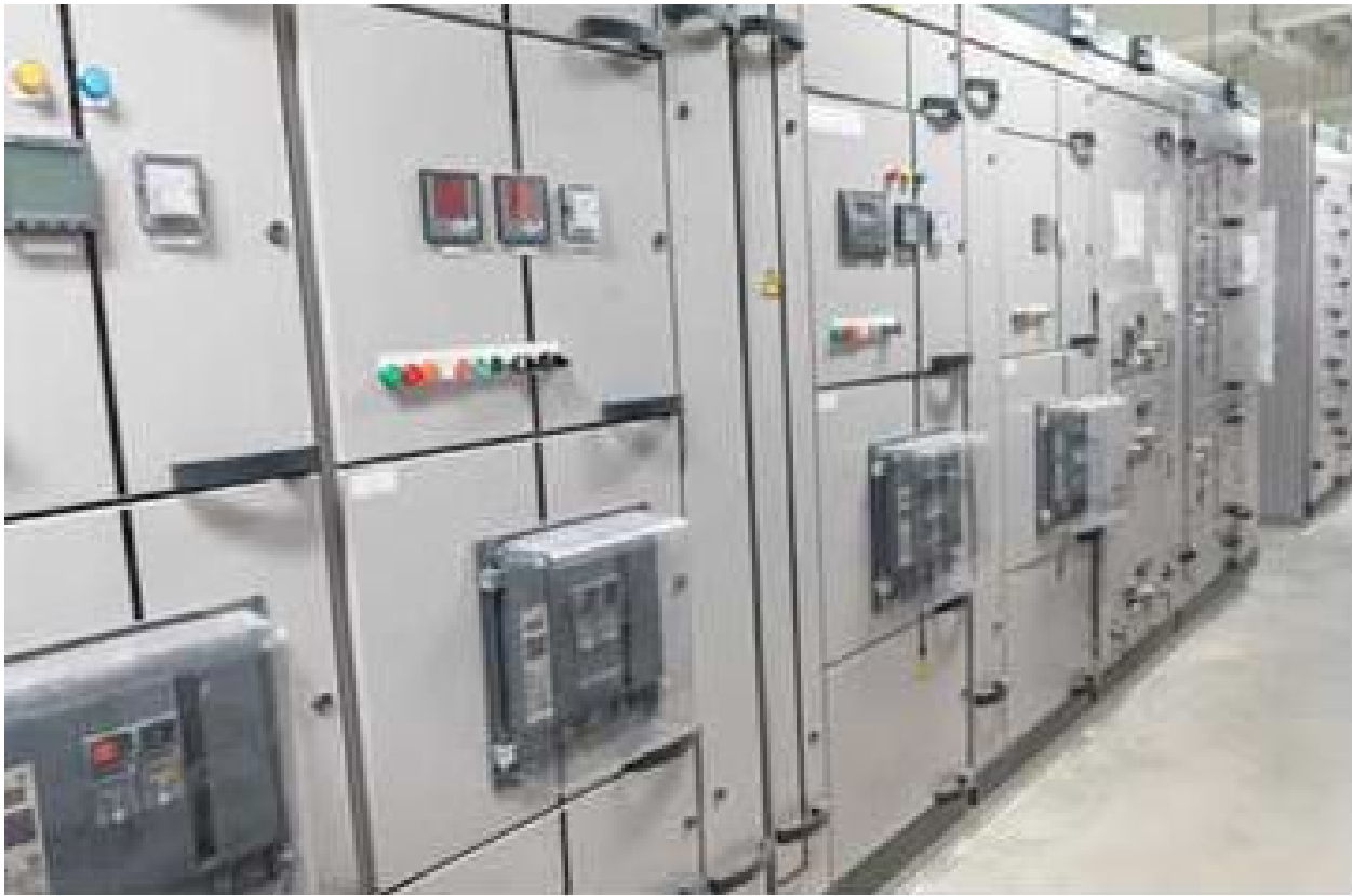
MOTOR CONTROL CENTERS
